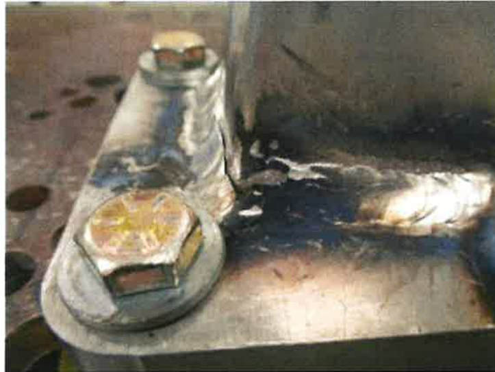
Photo No. 3 Typical Failure at Weld on Base Plate
